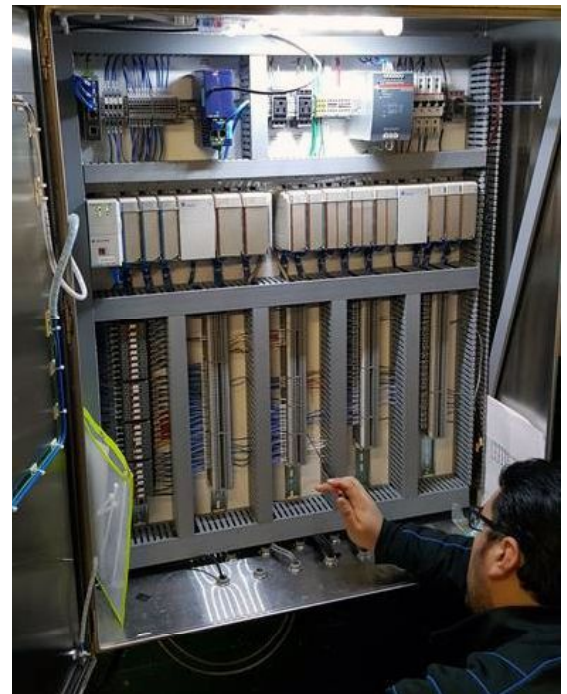
Allen-Bradley® PLC cabinet
