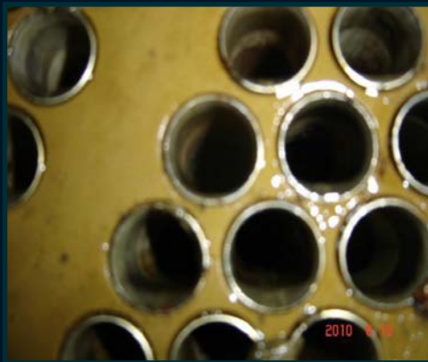
(June 2010) U15 Main Condenser Tube Sheet after extended run – before cleaning, after 2.5 Months of MIOX treatment
